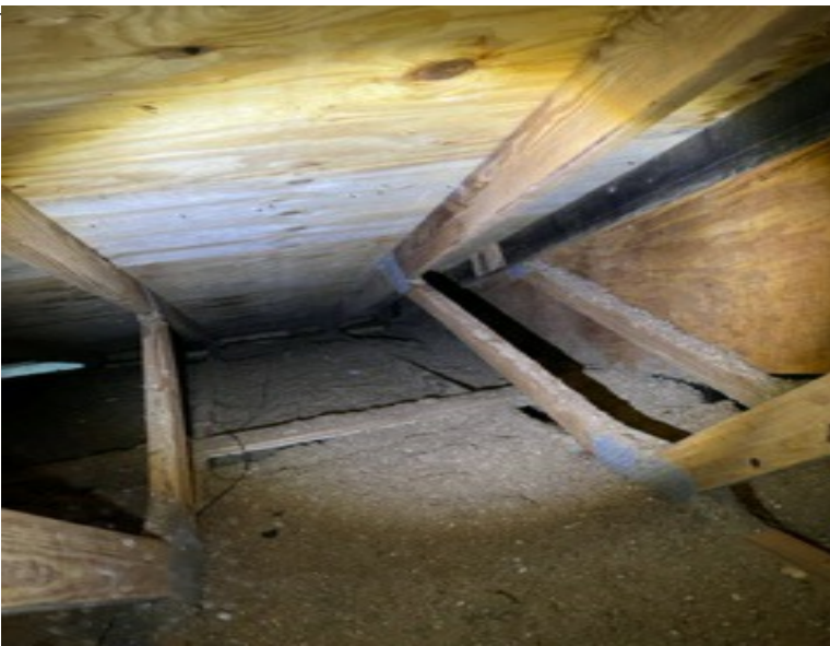
Active moisture found in several locations.
