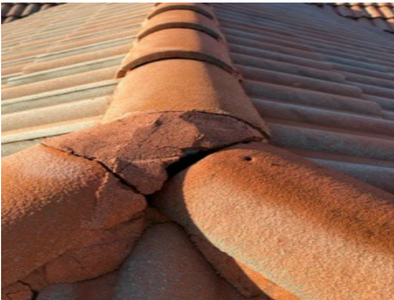
Mortar repairs needed in various areas.
