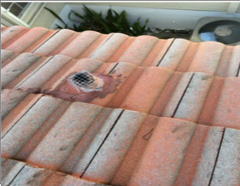
Cracked tiles and vents that need new mortar installed.
