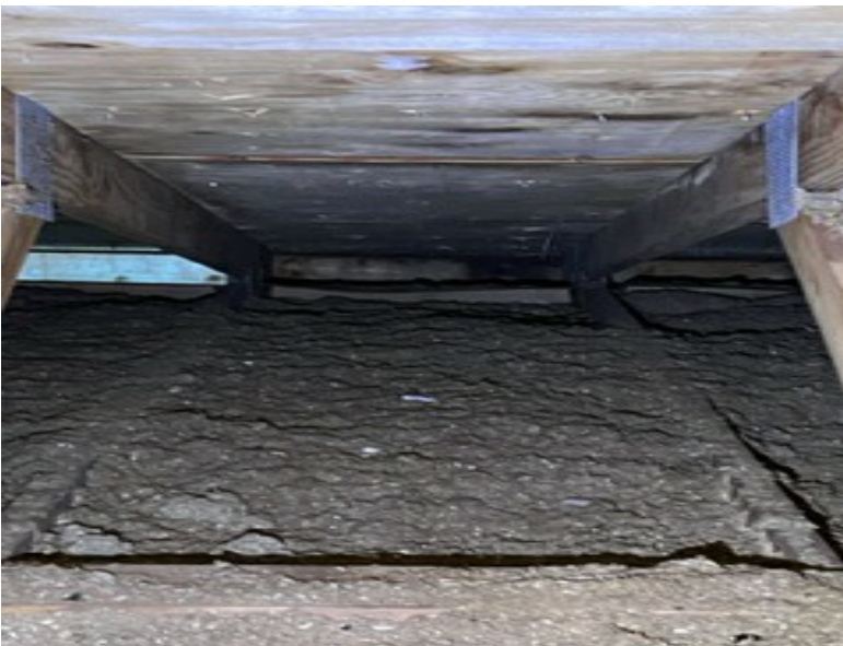
Active moisture found in several locations.
