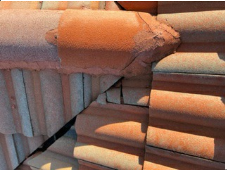
Areas that need new mortar installed.
