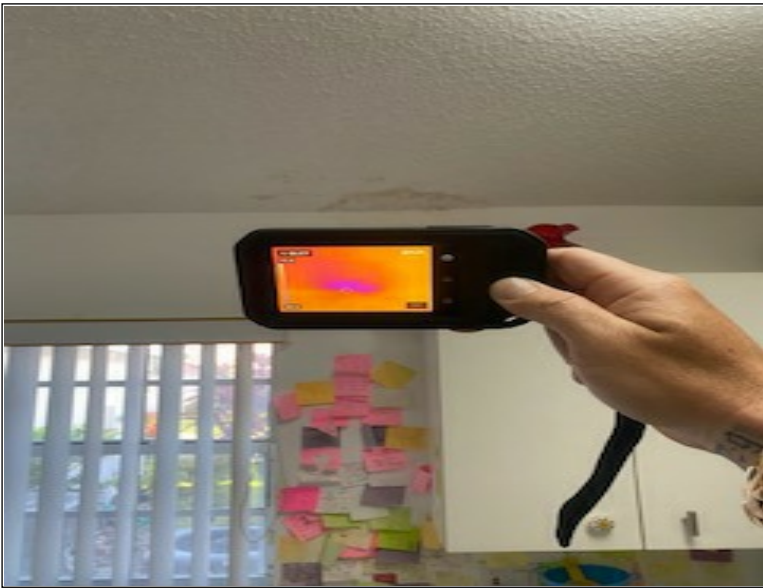
Active moisture found in several locations.
