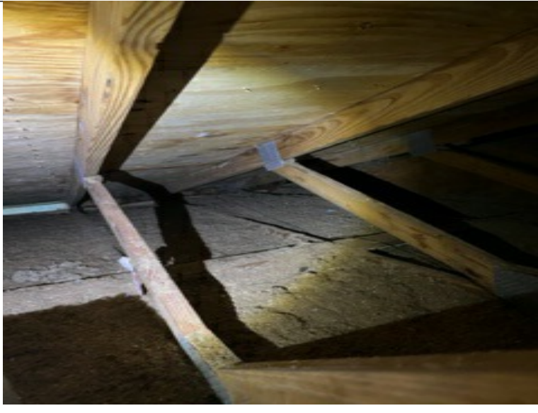
Active moisture found in several locations.
