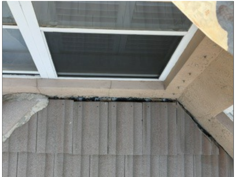
slipped and loose tiles across various sections of roof that need to be refastened.
