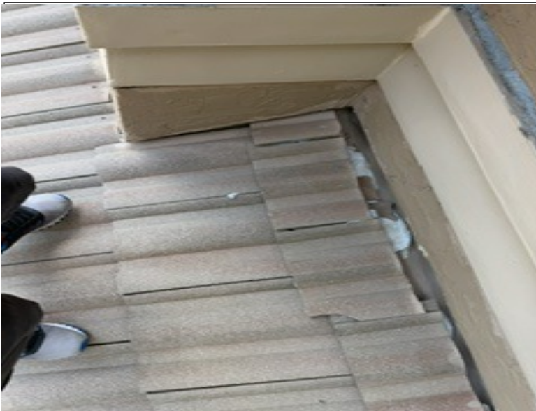
slipped and loose tiles across various sections of roof that need to be refastened.
