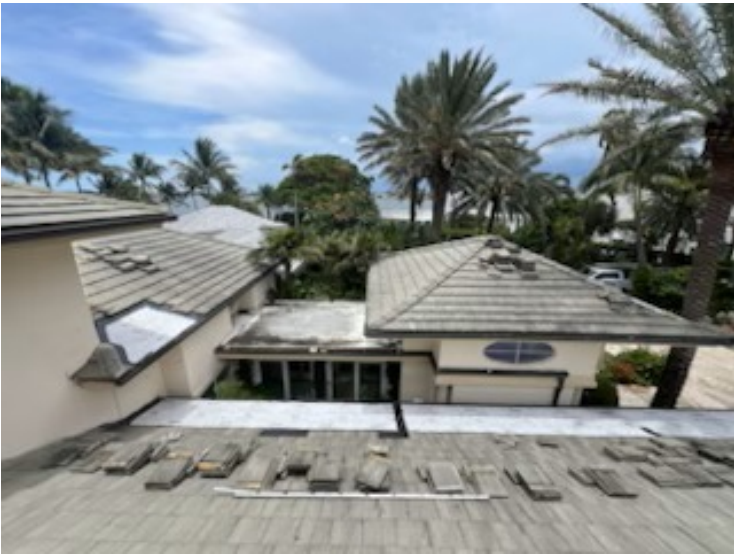
Roof section fully rebuilt with new plywood sheathing, underlayment, flashing components, and original roof tiles reinstalled to their original placement.
